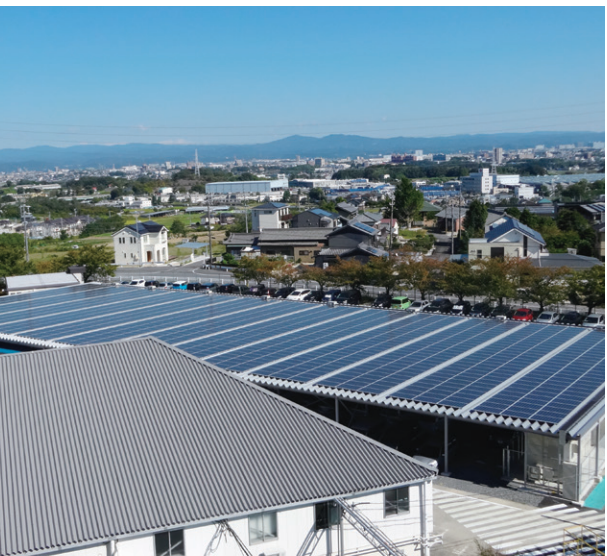
Solar power generation equipment (MIYOSHI SITE)
