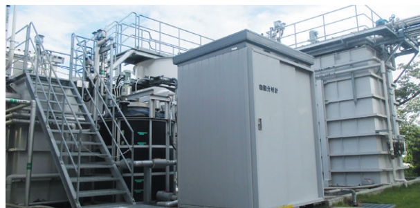
Wastewater processing equipment
